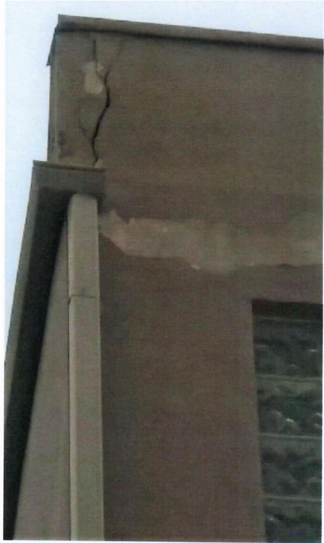
CRACK IN PARAPET WALL — FRONT TOWER
